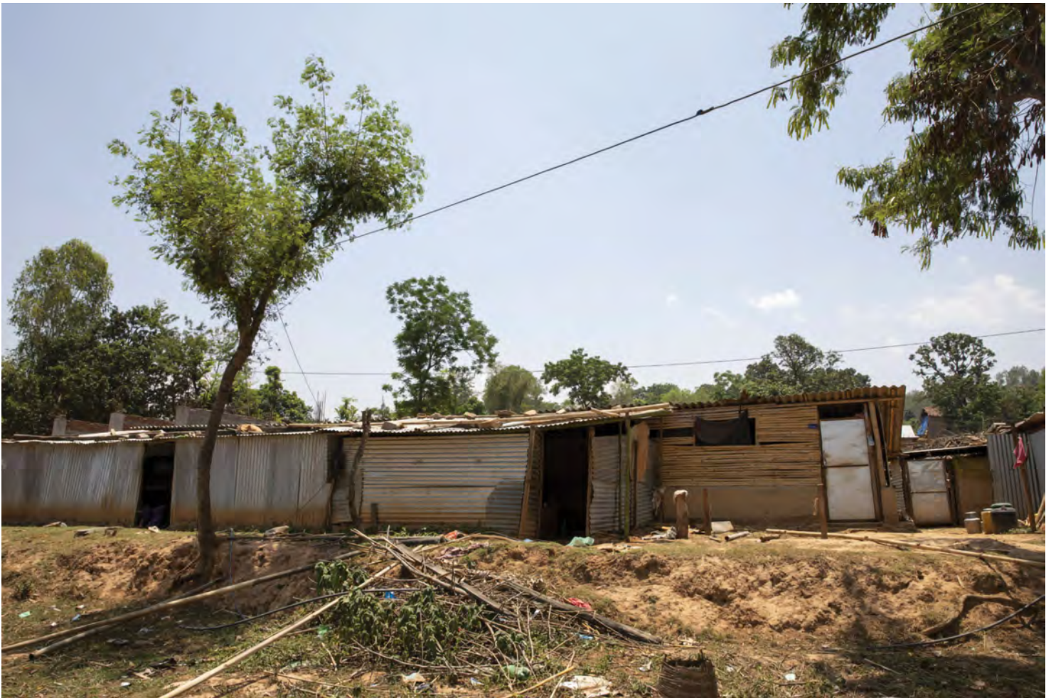
Many families in Nepal live in homes that are constantly on the verge of collapse.
